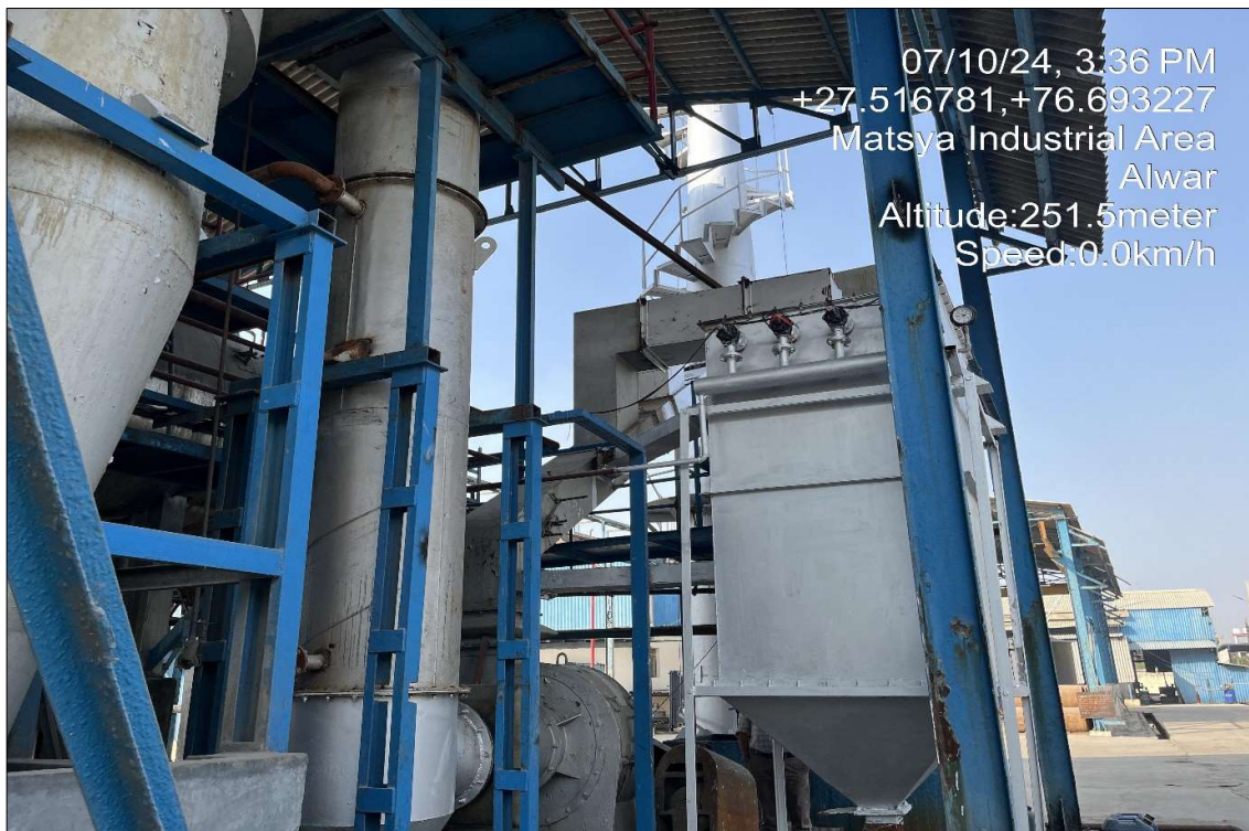
Fig 02: Emission control measures adopted at the boiler in M/s Ajanta Polymers Pvt. Ltd.
