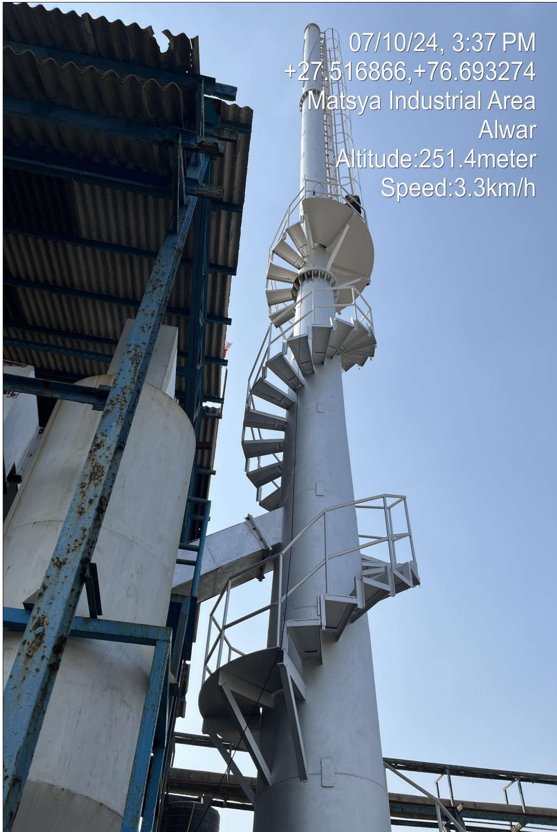
Fig 03: Stack of height approximately 30 meters has been provided with the boiler in M/s Ajanta Polymers Pvt. Ltd.
